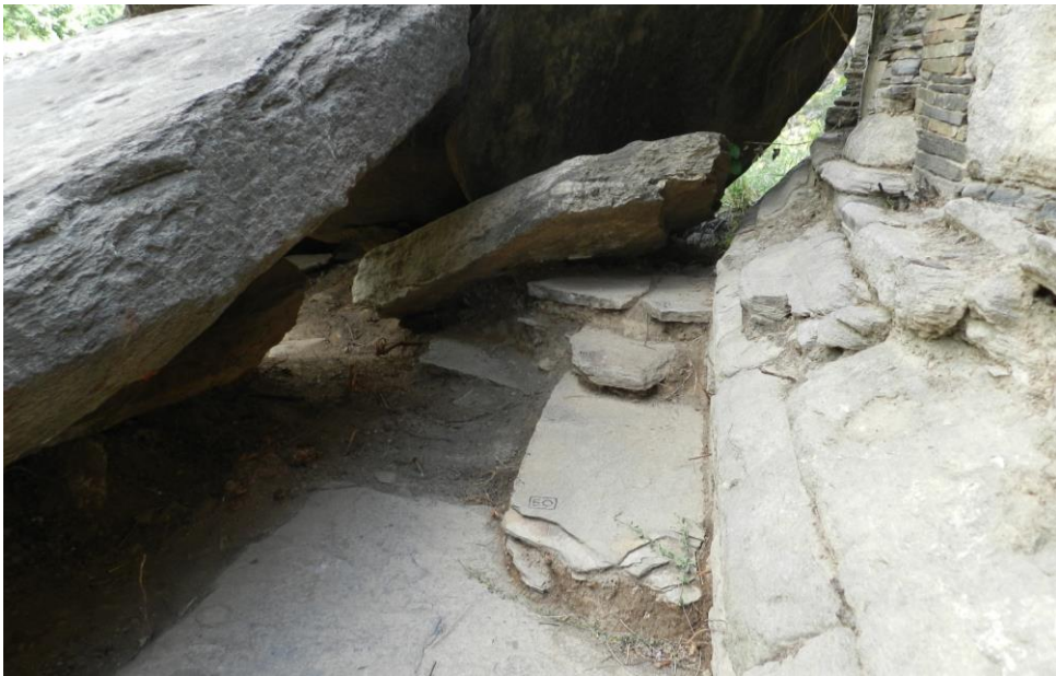
Figs. 30-31 - Two views of the chattras on the E side of the top floor of the podium. The picture above shows also the rows of brackets and coping that mark the upper storeys. In correspondence with the collapsed chattras, the row of brackets is missing. The left picture shows traces of four of the superimposing floors on the top of the 1st storey. (Photos by LMO).
