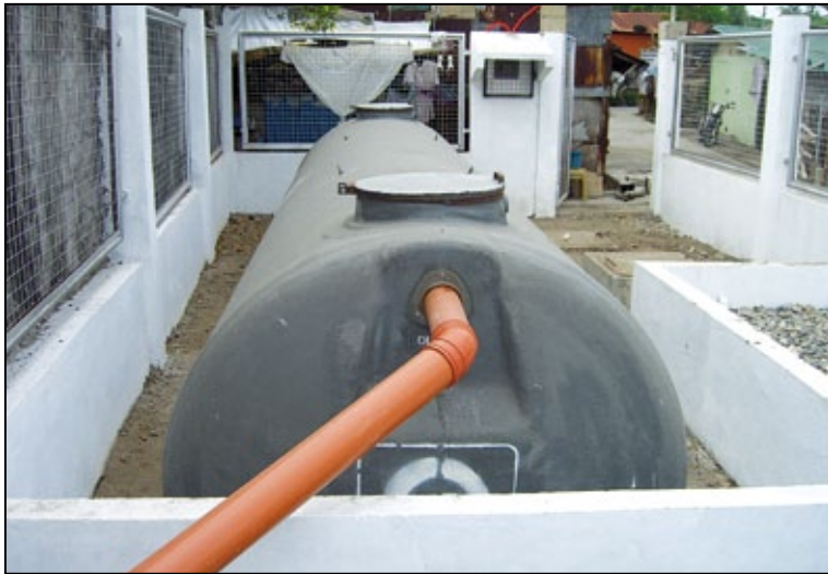
Figure 8: Eco-Tank installation completed in low-income riverside community
