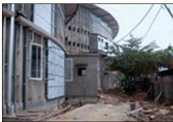
Figure 2: New bus terminal (target site) under construction in Negombo with Eco-Tank installation completed
