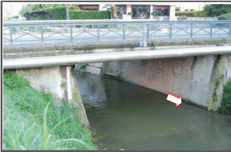
Figure 6 – Hydrometer at Borgo Vicenza bridge (Castelfranco Veneto)
