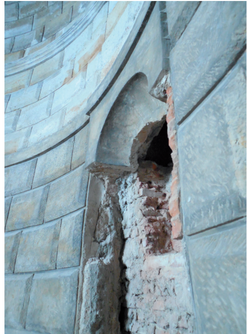
9. Prague, Bubeneč Grotto, ruined niche showing the thin surface layer of stonework
