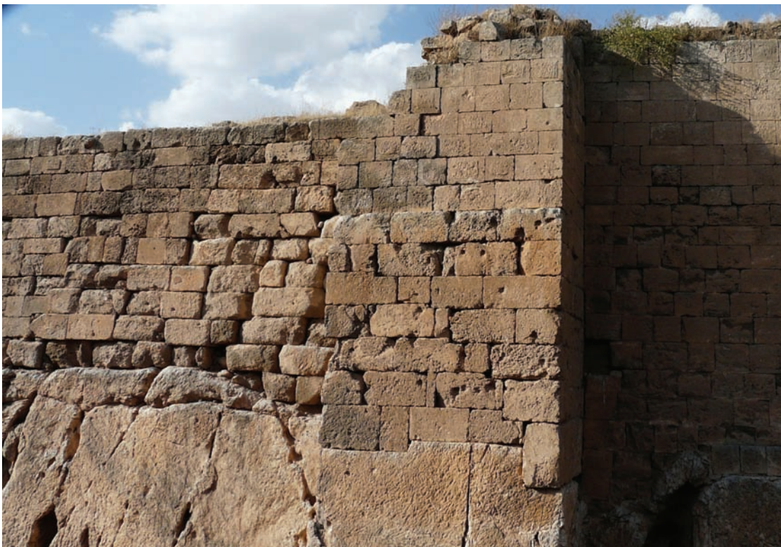
Fig. 4 – Buttress T8, from the South. The lower part belongs to Period 2 (©C. Tonghini)
