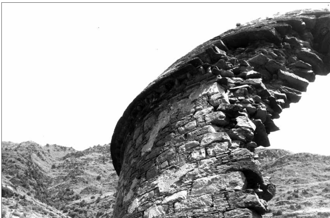
Fig. 521. Gumbatuna, Vihara. SW side; upper part of the outer wall of the cell showing remains of plaster, cornice and the beginning of the dome. (Faccenna 1960; Neg. CS).
