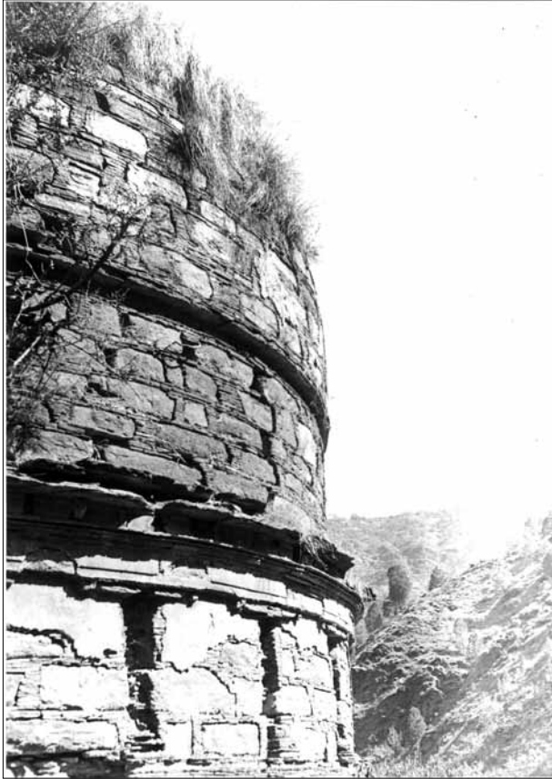
Fig. 297. Abbashehchina. Stupa C. E side, 3 rd , 4 th and 5 th storey with socket lacking projecting slabs; profile. (Taddei 1957).
