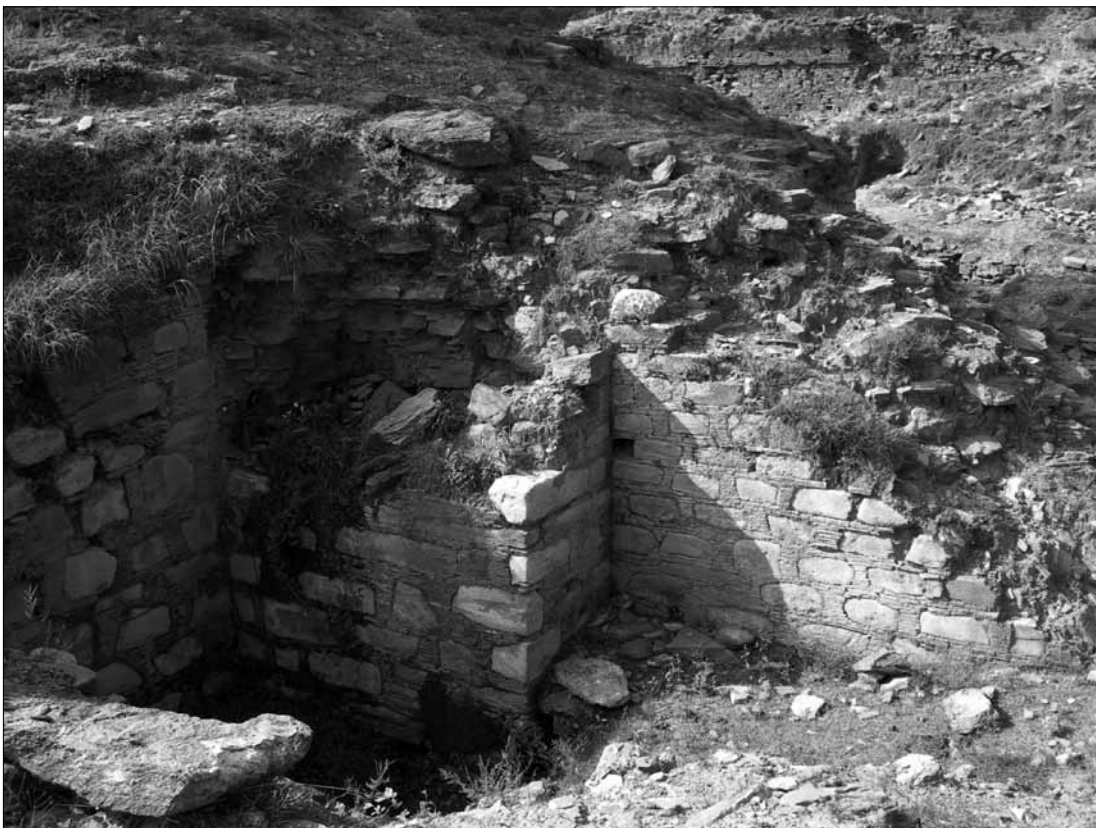
Fig. 342. Stupa of Tokar Dara (Najigram). 1 st storey, W side, N side of the stairway with projection; detail. (Spagnesi 2005).
