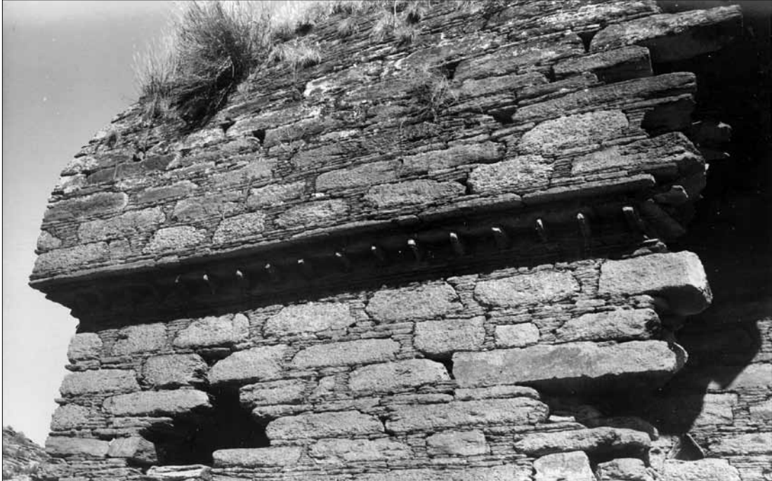
Fig. 465. Vihara of Gumbat. S side; cornice of the lower roof covering. (Taddei 1959; Neg. CS).
