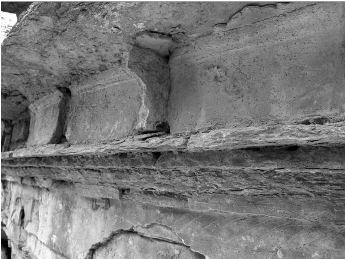
Fig. 302. Abbashehchina. Stupa C. SE side, 3 rd storey; modillions of pilasters, stretch of architraved and bracketed cornice; plaster remains. (Spagnesi 2005).
