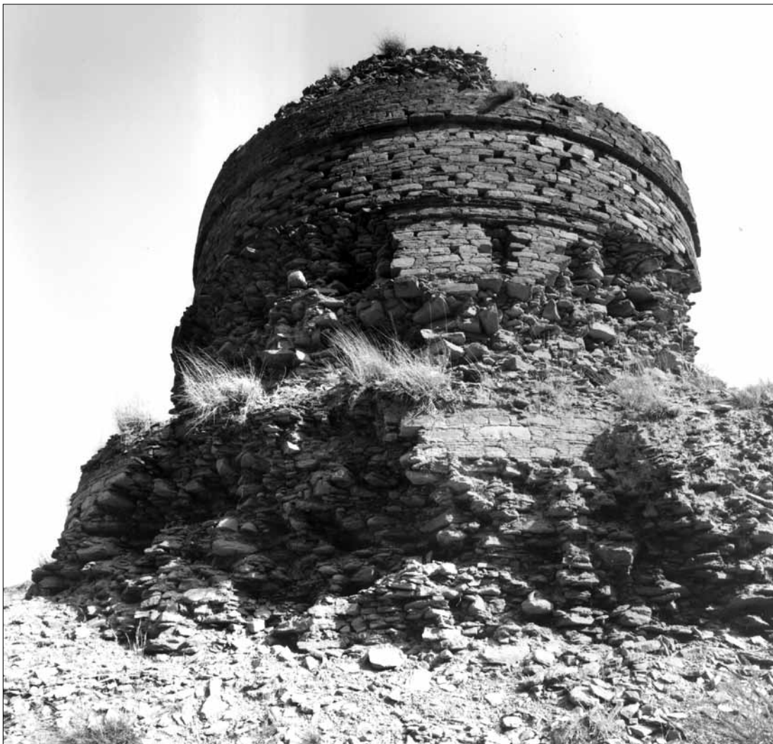
Fig. 392. Stupa of Top Dara (Haibatgram, Thana). SE side; 4 th and 5 th storey and remains of the 3 rd storey wall. (Kuwayama 1993).
