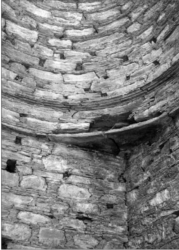
Fig. 447. Abbasahebchina, vihara F. Inside the aedicula (B); dome springer lying on slabs; detail of SW side with corner slabs and overlying band (F, G). (Taddei 1957; Neg. CS).
