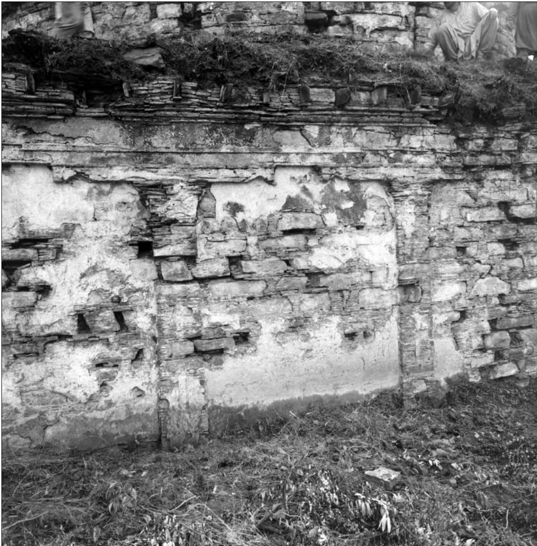
Fig. 234. Abbasahbchina. Stupa A. N side, 1 st storey, with remains of plaster. (Kuwayama 1993).
