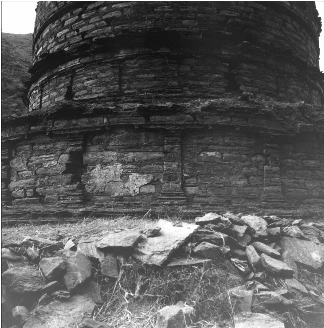
Fig. 239. Abbasahebchina. Stupa A. S side, 2 nd storey, with remains of plaster; 3 rd storey (drum) and 4 th storey (transition storey of the composite dome). (Kuwayama 1993).
