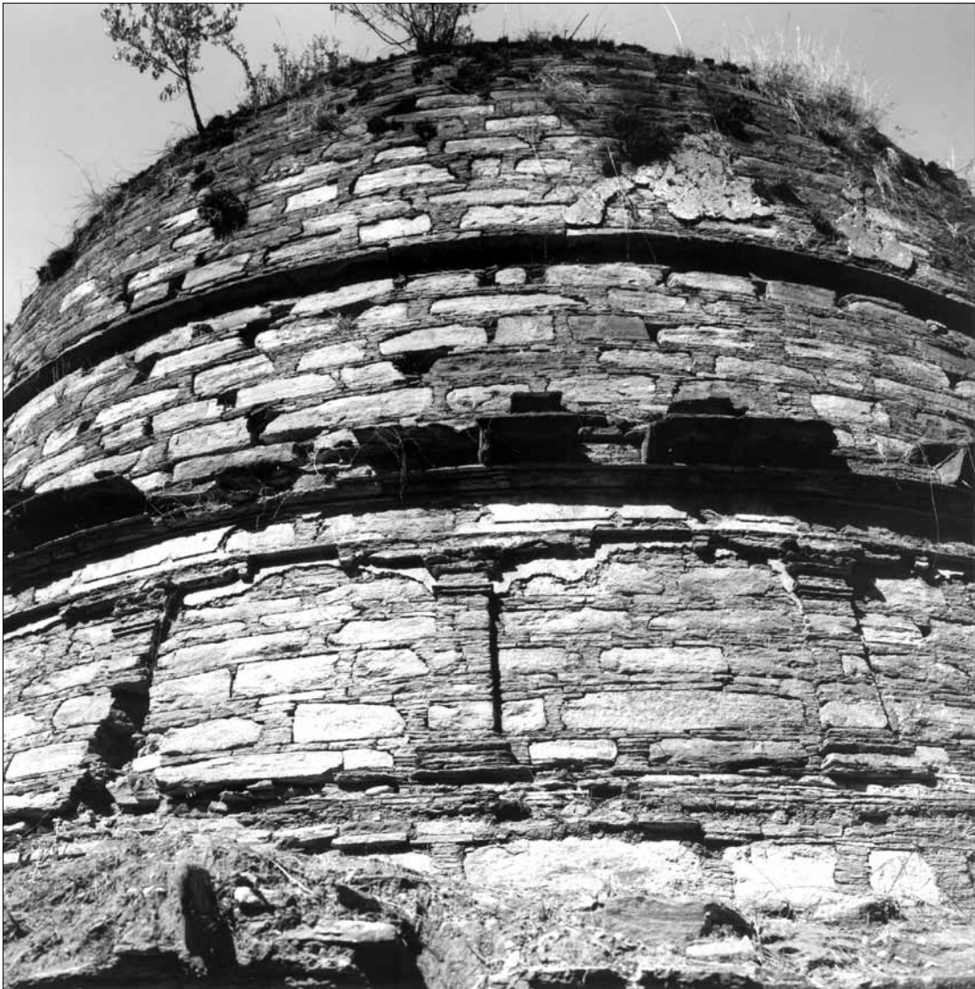
Fig. 240. Abbashehchina. Stupa A. Lato SE side, 3 rd storey (drum), 4 th storey (transition storey of the composite dome), 5 th storey (raised dome); with remains of plaster. (Kuwayama 1993).
