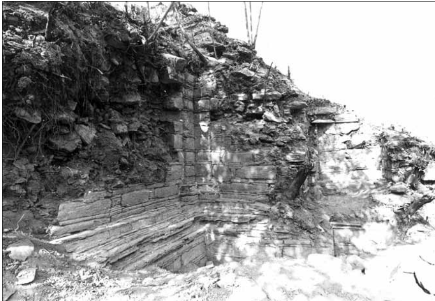
Fig. 52. Stupa of Loebanr. 1 st storey, S side. A stretch of the storey, projection with inner corner pilasters, stairway, cell; at the top, stretch of the stairway of the 2 nd storey. (Nascari 1993; Neg. CS).
