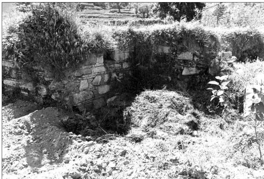
Fig. 50. Stupa of Loebanr. N-S substruction wall of the Monastery on the W side of the Stupa. (Nascari 1991; Neg. CS).
