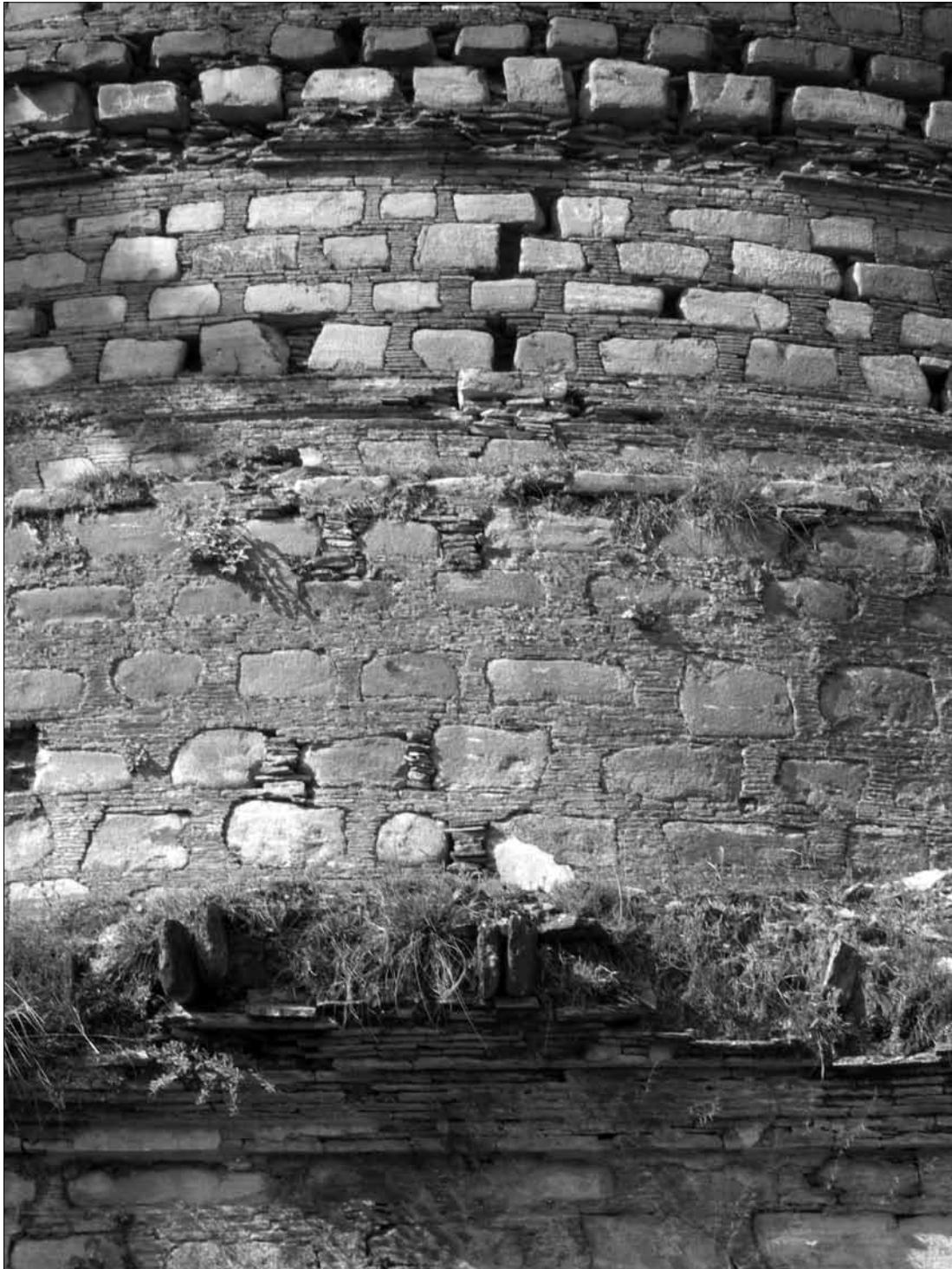
Fig. 349. Stupa of Tokar Dara (Najigram). N side, 1 st , 2 nd and 3 rd storey showing visible stretches of the bases and cornices. (Spagnesi 2005).
