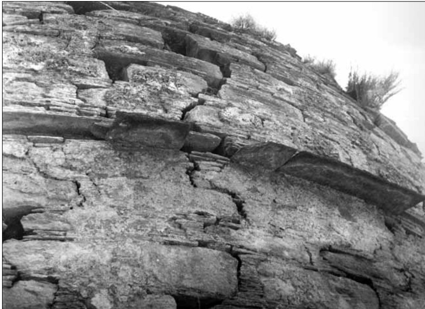
Fig. 299. Abbasahebchina. Stupa C. E side, 4 th and 5 th storey with socket with projecting slabs. (Taddei 1957; Neg. CS).
