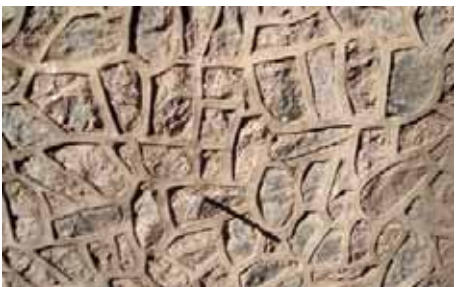
4. Cracks in the stone masonry facade
