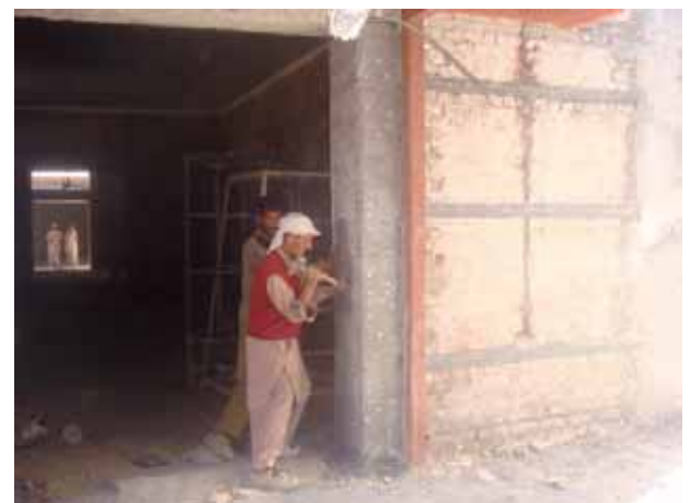
25. Wall stitching and RC column connection. Wire mesh is also visible
