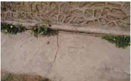
5. Crack in the plinth protection
