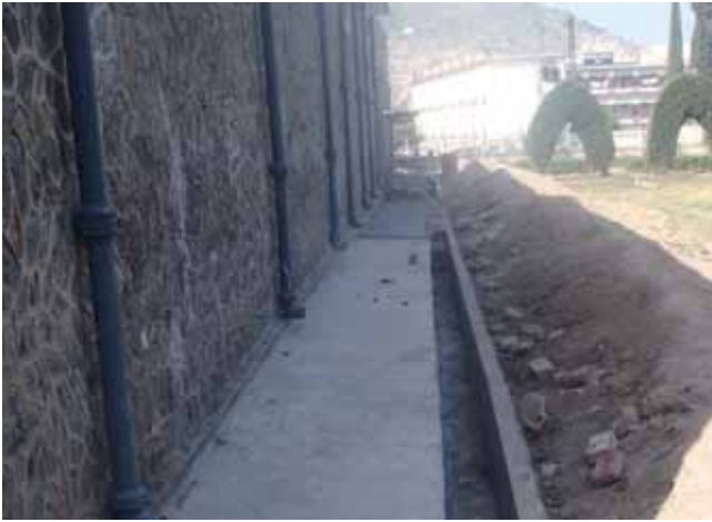
26. Plinth Protection and drains in old block
