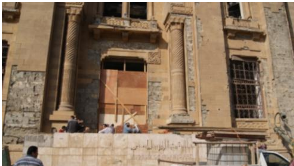
Figure 13: The main door of the museum and part of the façade after the blast ( photo :Museum of Islamic Art )
