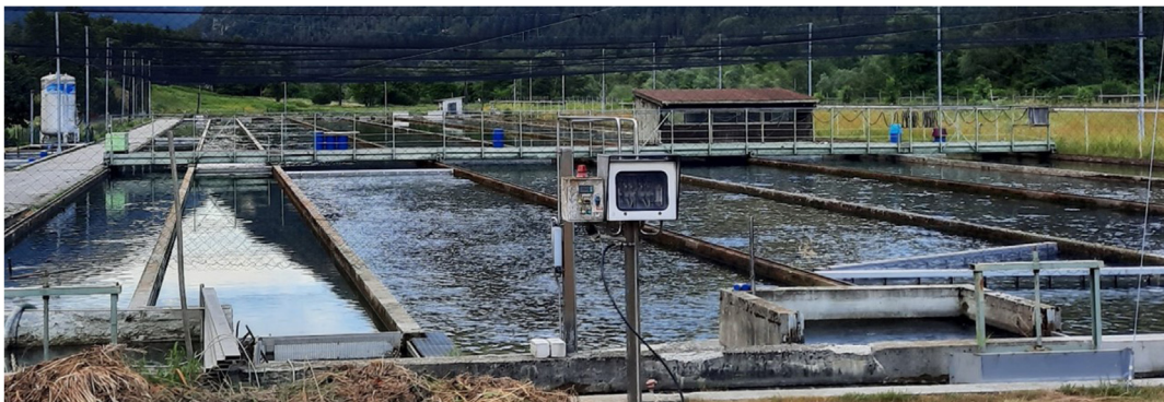
Figure 1. Raceway tanks, the liquid oxygen tank (white tank in the left) and the gantry (containing movable catwalk which crosses the raceways).
